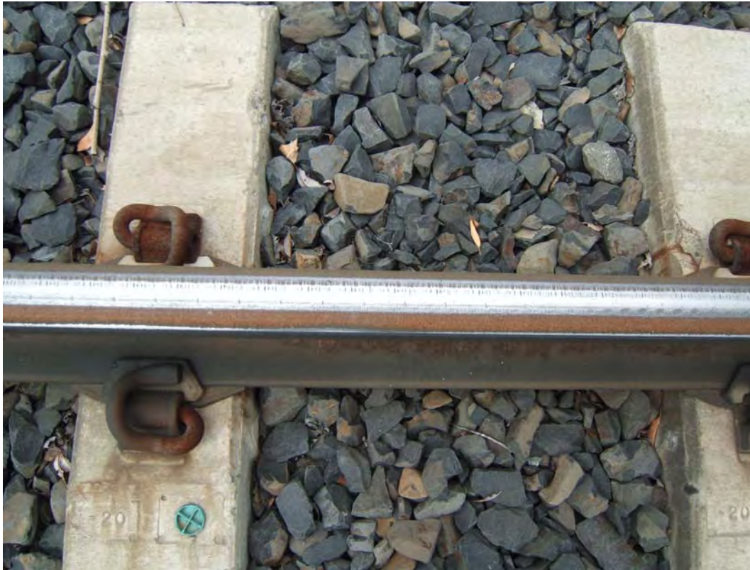
FIGURE 6 - RAIL CONDITION AT SITE 1
