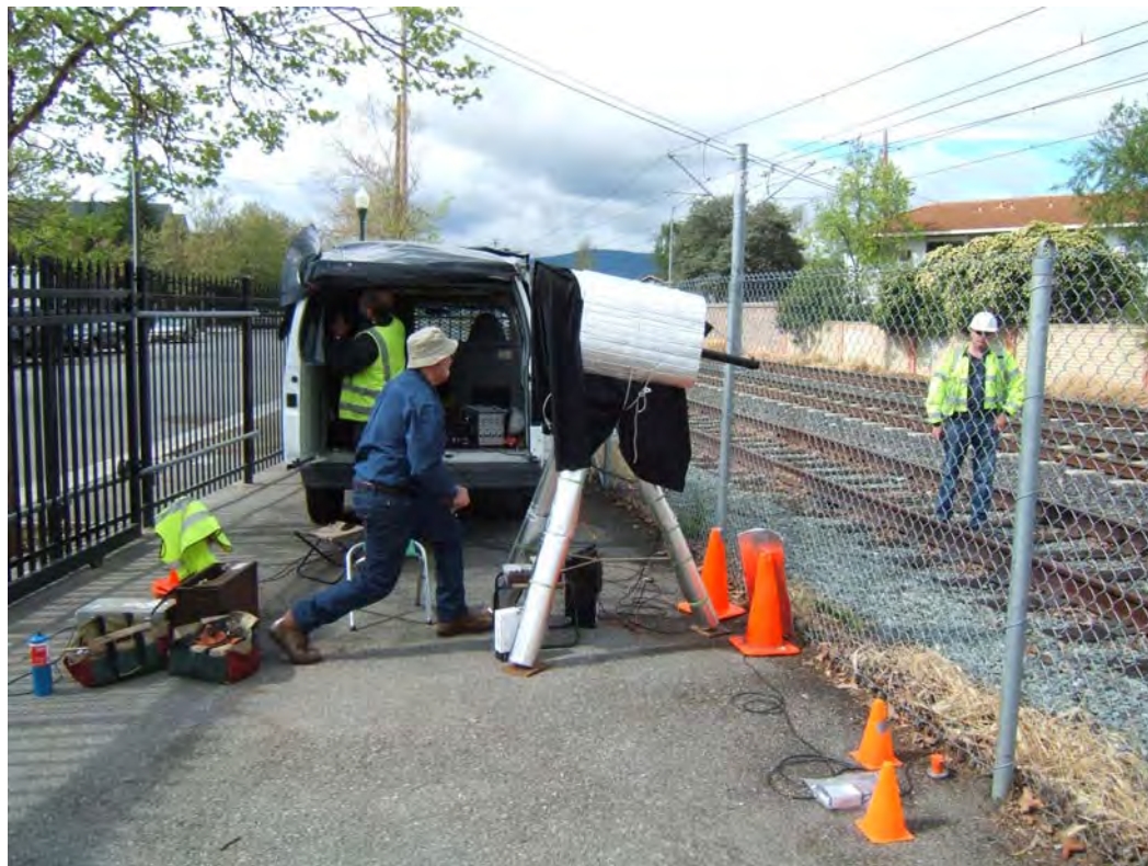
FIGURE 5 - OPTICAL RAIL DEFLECTION MEASURE DEVICE AT SITE 1
