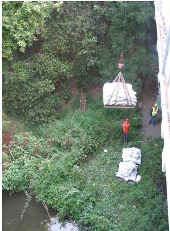
Figure 11 – Photo of Sand Bag Crane Operation. Sand bags being landed on north side of bridge between Pier Nos. 2 and 3.
