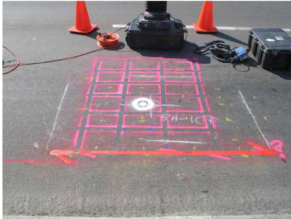
Figure 8 – Photo of Marked Deck Reinforcement Locations. GPR equipment in background. Photo taken from north curb looking south.
