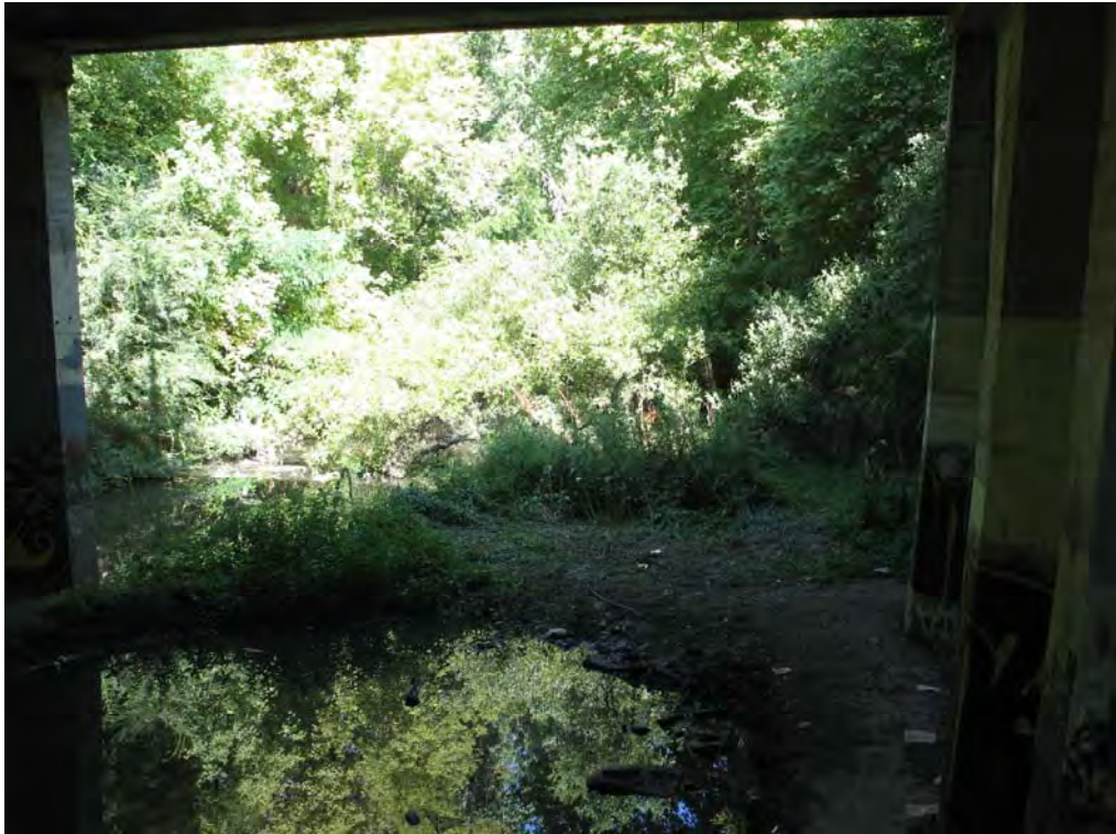
Figure 14 – Photo of Restored Work Area Beneath Bridge. Stinging Nettles in landing area have been flattened by sandbag pallets. Pier No. 3 to right, photo is looking northwest.
