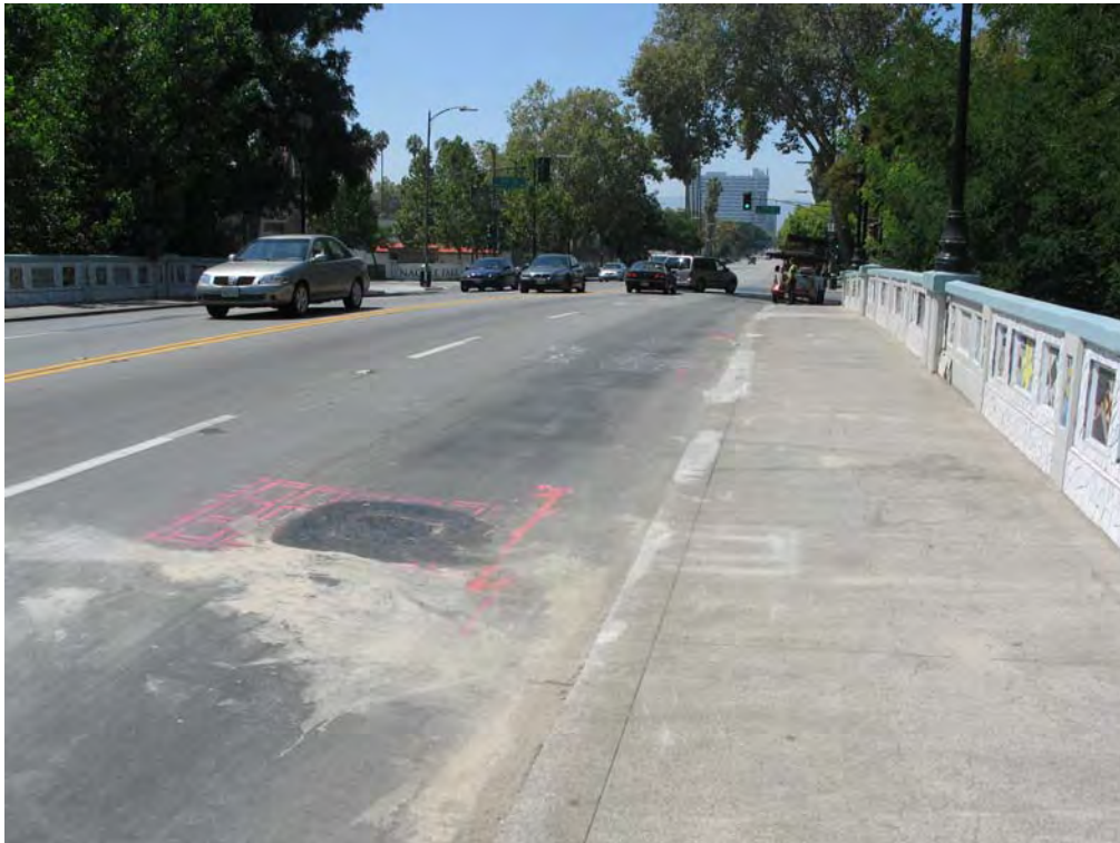
Figure 17 – Photo of Completed and Restored Bridge After Work Completion. Photo looks southwest.
