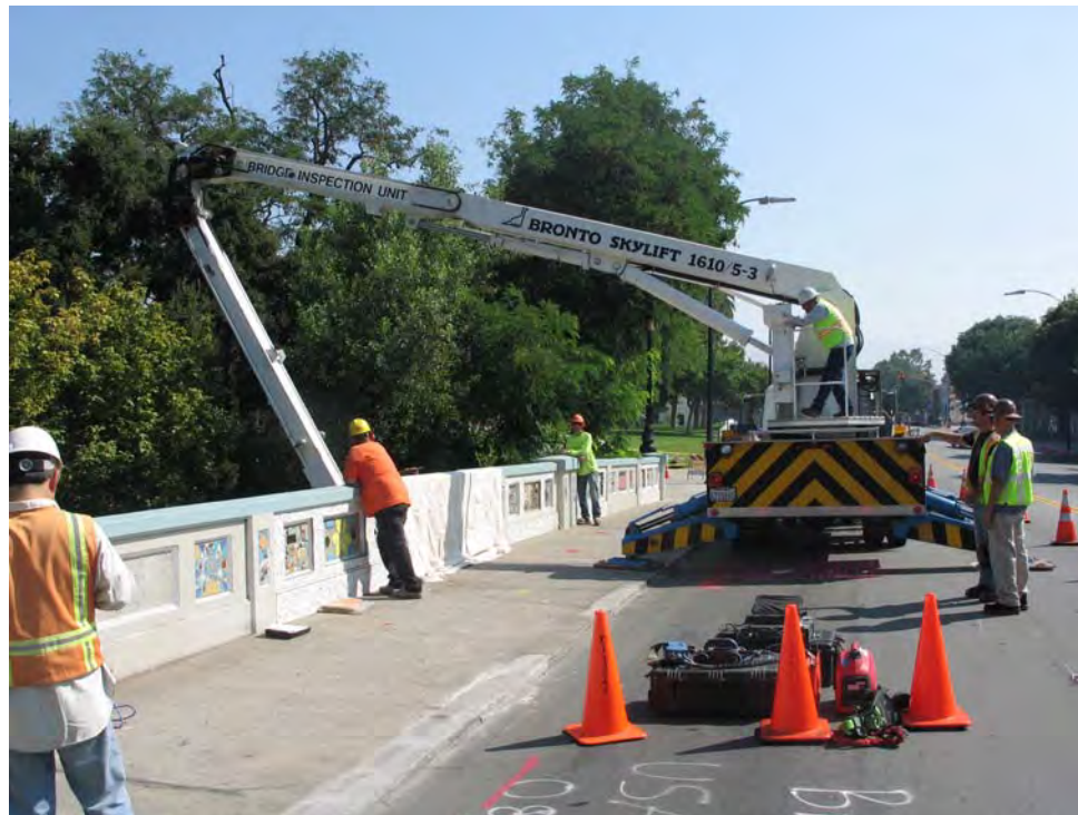
Figure 9 – Photo of bridge inspection truck. BH-107 is located under the aft of the inspection truck. Access to the base of the deck could not be achieved with this equipment.
