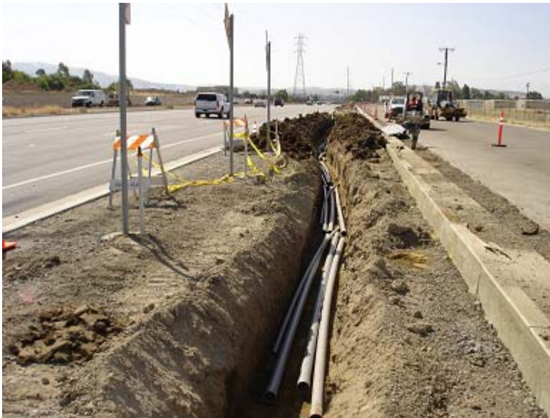
Conduit for lighting and bus stop
