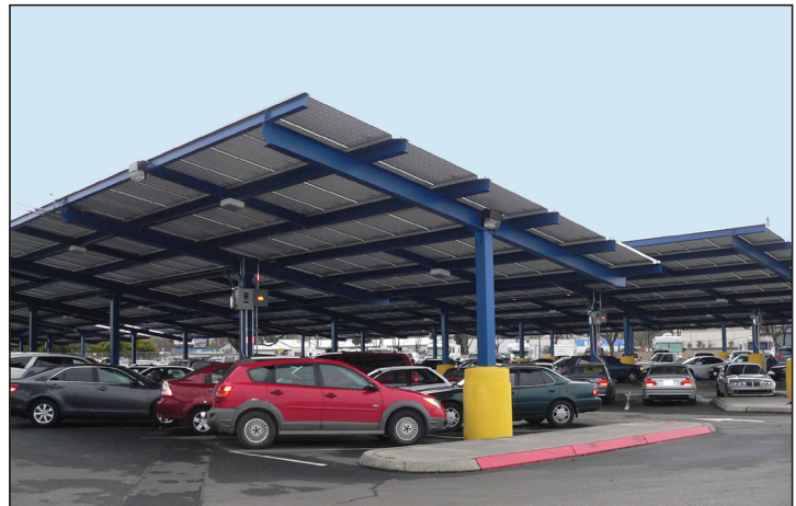
Employees park under the solar canopies at VTA's Chaboya Maintenance Division, 2240 South 7th Street in San Jose.
