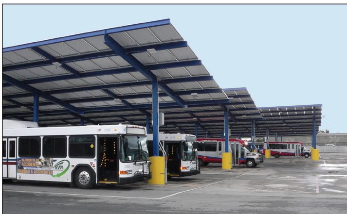
Buses utilize parking for shade and weather protection underneath the solar canopies at VTA's North Maintenance Division, 1235 La Avenida Street in Mountain View.
