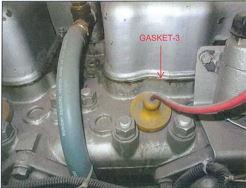
Photo 13: Generator Exhaust Manifolds
