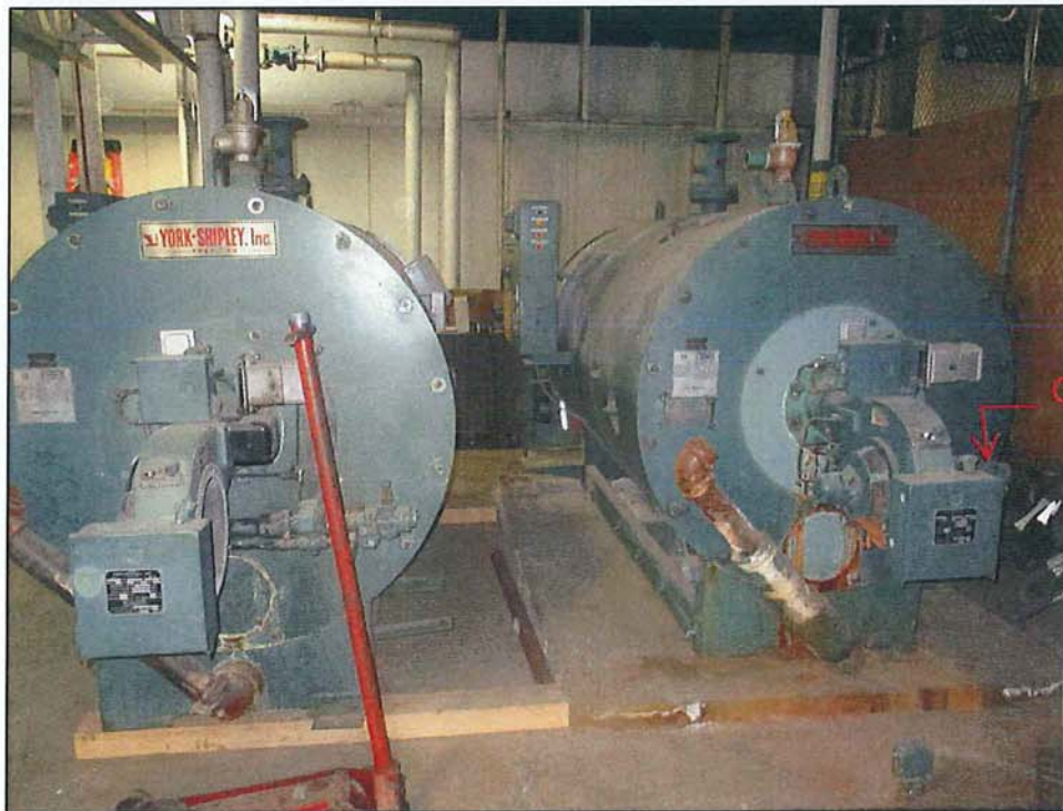
Photograph 14: Gasket-17: on Fan Assemblies of Boilers
