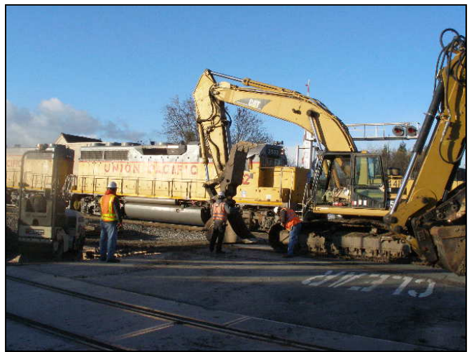
Replacement of existing Dixon Landing Road grade crossing of UPRR Main Track 1
