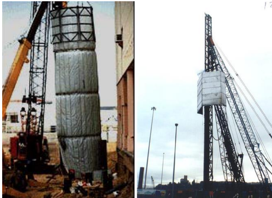
Figure 13: Impact Pile Noise Shrouds. Image on the left shows an effective enclosure. Image on the right shows a marginally effective barrier.
