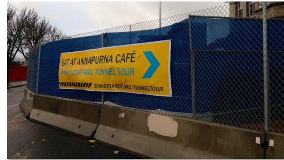
Advertisement for local business during construction of Capitol Hill Light Rail Station – Sound Transit
