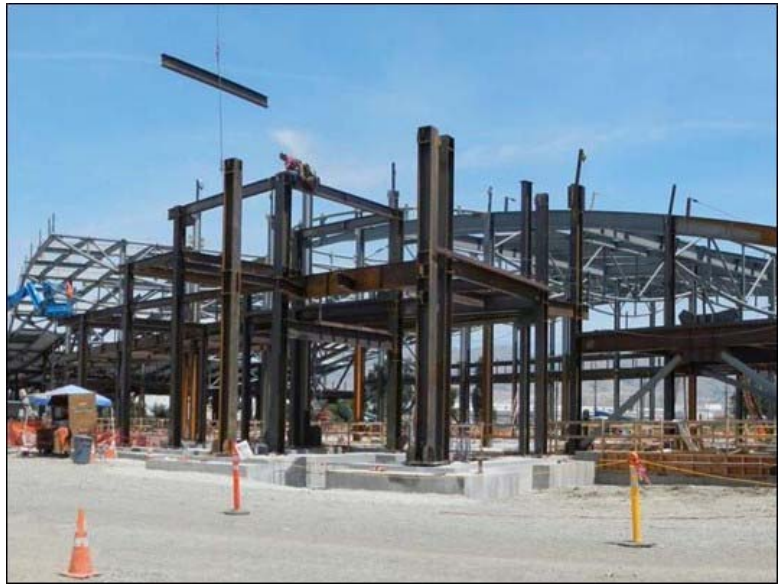
Installation of Steel for the Pedestrian Overcrossing at the Milpitas BART Station
