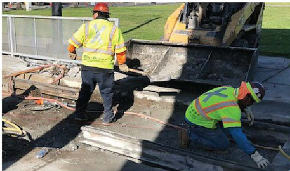
VTA performing Rail Rehab to keep our light rail system in shape
