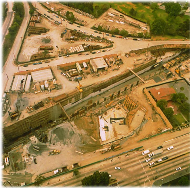
LA Metro – Universal City Station Excavation (similar site constraints as Alum Rock)
