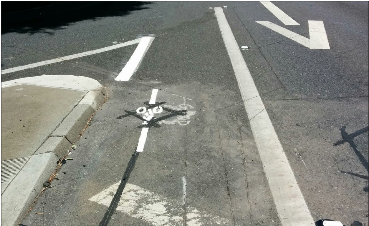
b. View of a bike detector embedded in a bike slot. The purpose of a bike detector is to detect a bicyclist approaching an intersection and communicate with the traffic signal cabinet to provide enough time for cyclists to safely cross an intersection.
