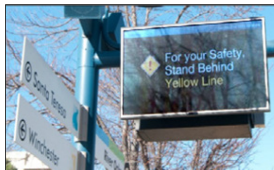
One of the many light rail platform passenger information signs installed this year.
