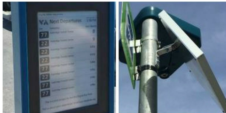
VTA's new solar-powered real-time information (RTI) signs
