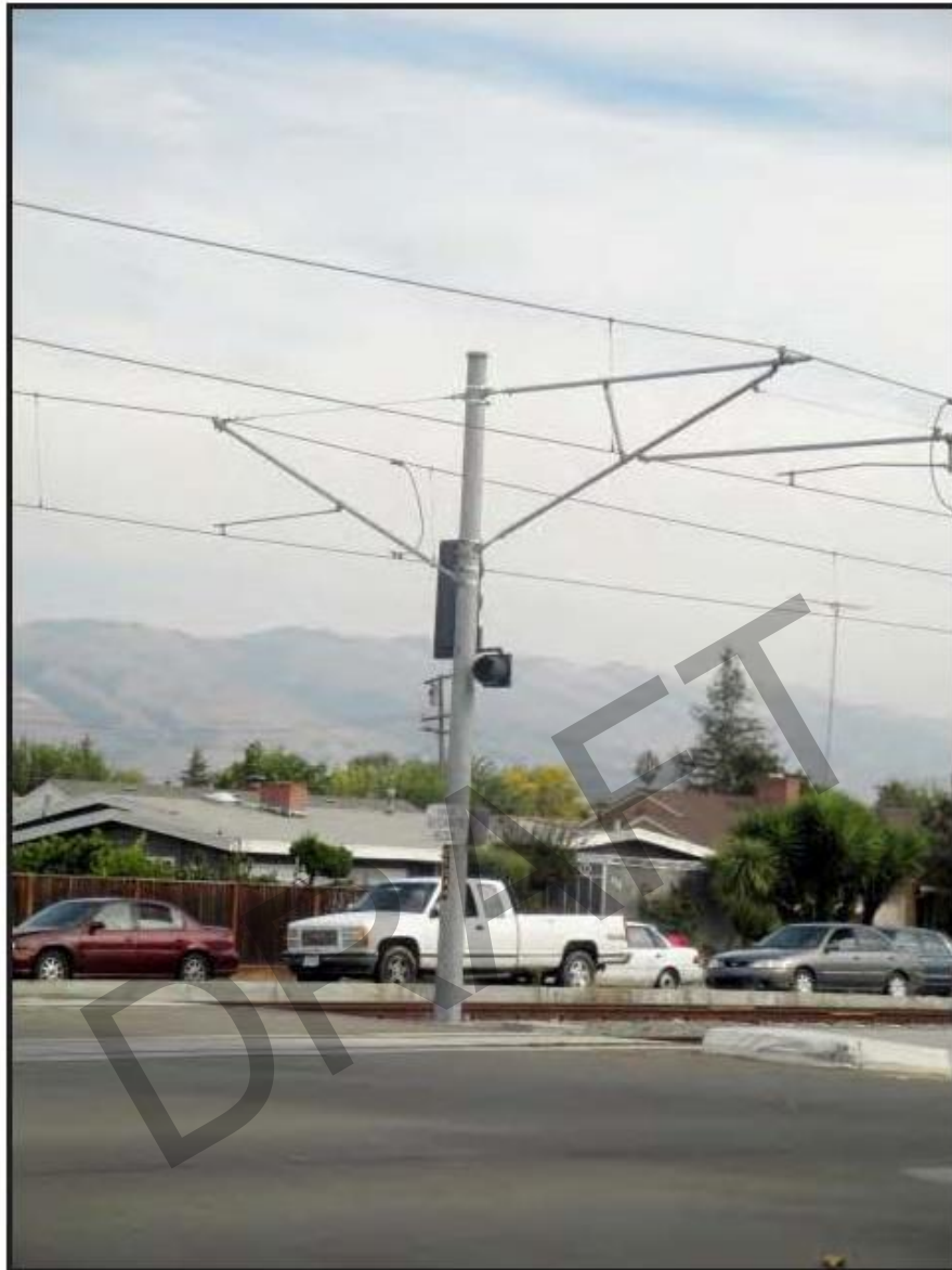
Figure 4 Overhead Contact System at Alum Rock Station
