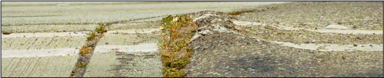
Asphalt bulge at end of bridge deck
