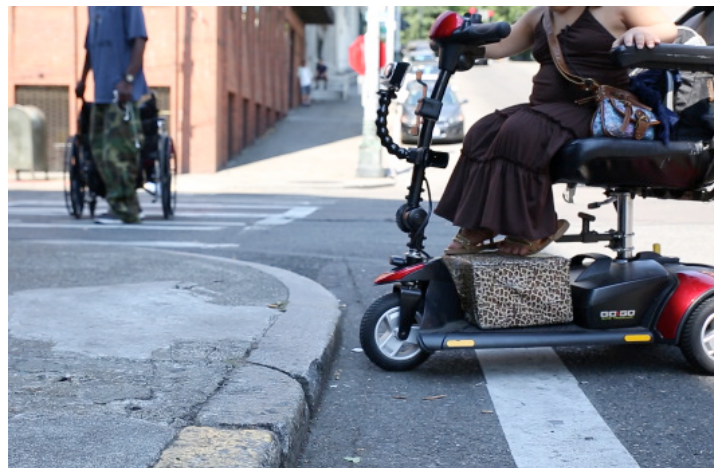
Missing Curb Ramp - Photo Credit: Disability Rights Washington
