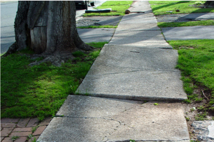
Broken sidewalk - Photo Credit: Medium
