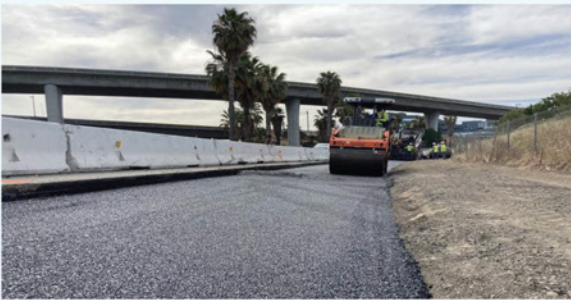
2016 Measure B funded the US101/De La Cruz Boulevard/Trimble Road interchange. New overcrossing was constructed to replace an existing 60 year old bridge.
