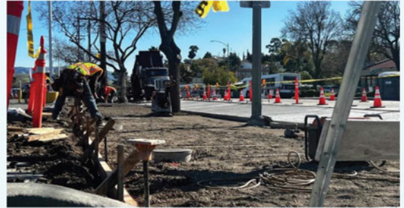
With the Better Bus Stop Program, VTA installed over 150 benches and new solar lights. Construction is ongoing for new shelters, bike racks, benches and sidewalk improvement.
