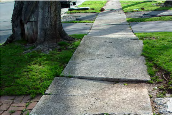
Broken sidewalk - Photo Credit: Medium
