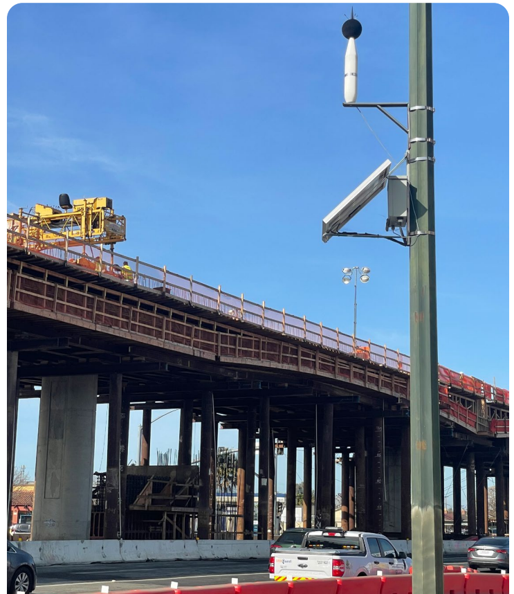
Noise and vibration monitors installed along the construction zone allow the EBRC team to ensure the project is in compliance with the Federal Aviation Administration. (Photo by Lupita Franco Peimbert).
