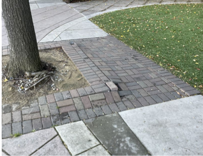
Uneven Paving at Great Mall Station Plaza
