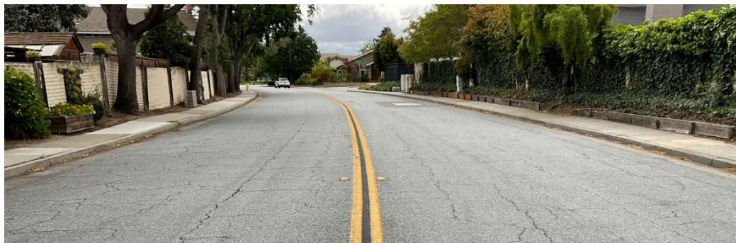
Pavement condition of White Oaks Avenue in the City of San Jose (Before)
