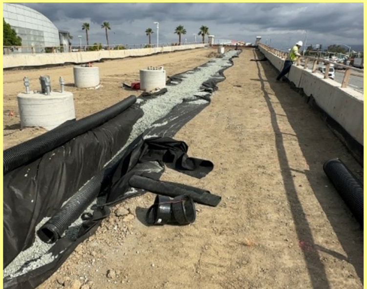
In this area the track sub drain is located within the ramp in the future VTA Eastridge Station.
